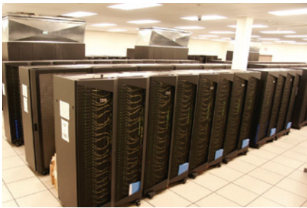
SciNet Data Centre
